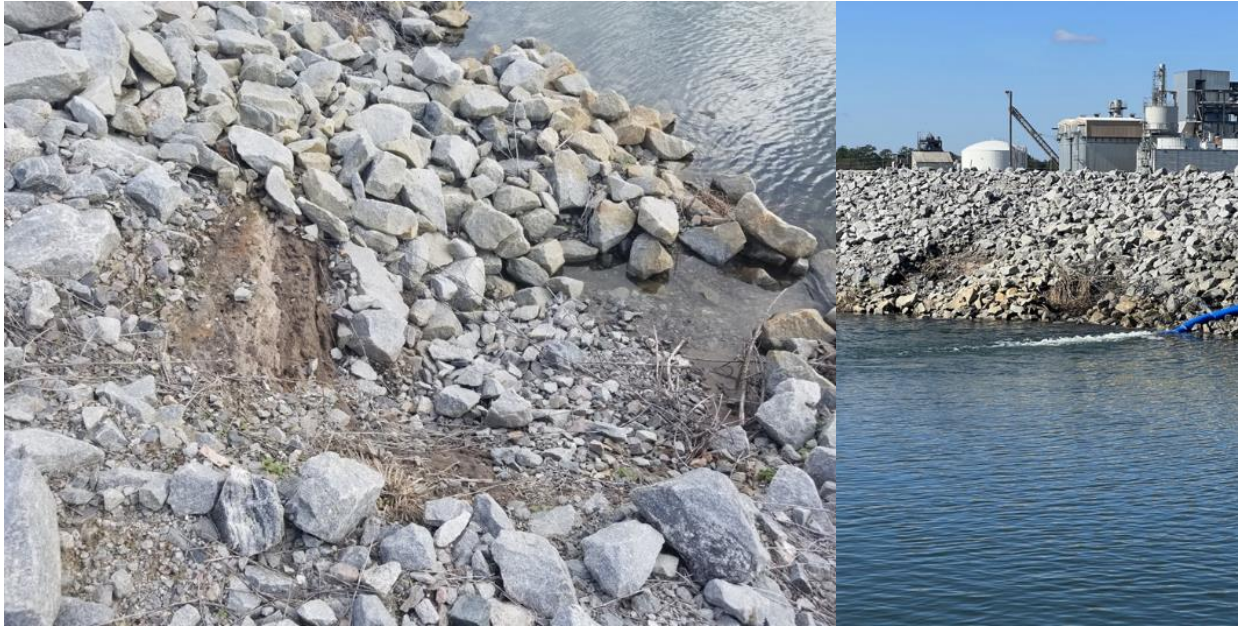
Figure 5. Ash Cell # 2 and Pump Back Cell #2 Embankment Erosion and Riprap Displacement
